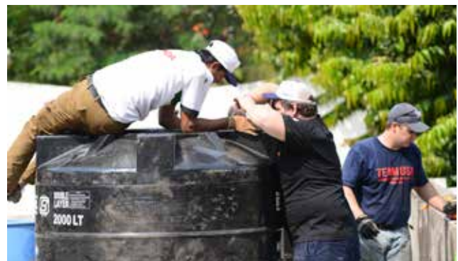
Members of Team India (Lalit Kasawate), Team Australia (Aaron Bridger), and Team USA (Adam Koenigs) work together on the school roof to install a new water tank that will supply the upgraded handwash area. Credit: Anill Patil
